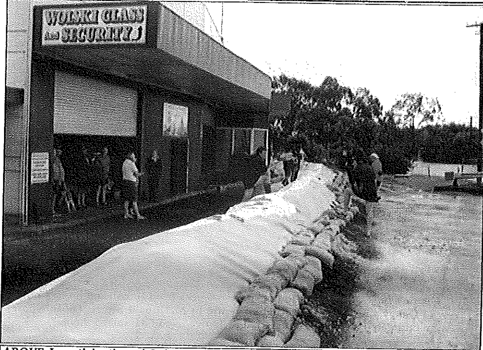
ABOVE: In anticipation of Oakey Creek topping the bridge, volunteers helped staff and owners to create a levy aimed at protecting the business.
