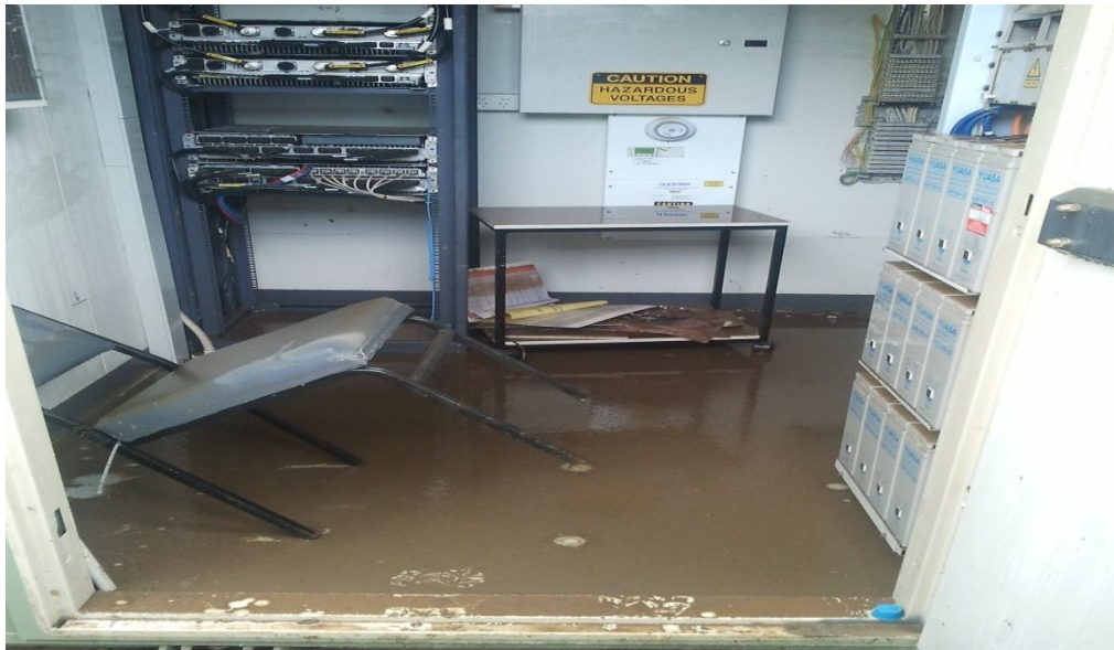
Picture: A water damaged Optus mobile base station, 2011
