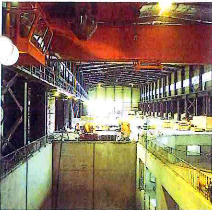
The 350-tonne travelling bridge crane ready for work over the equipment hatchway on the top floor.
