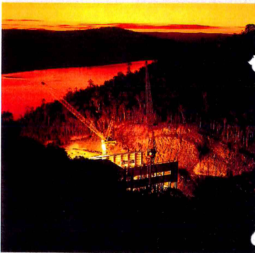
Wivenhoe Power Station at sunset.
