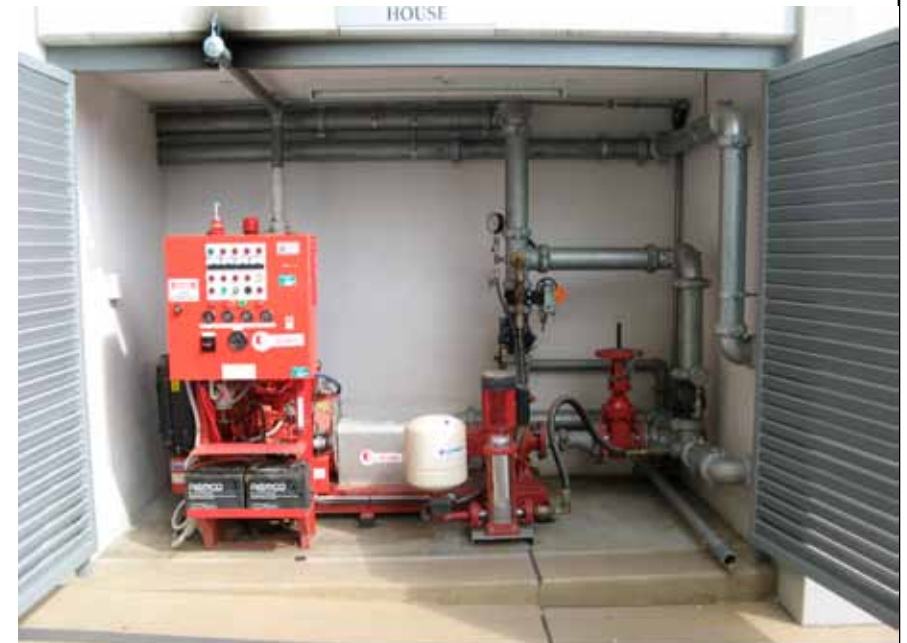
Main fire sprinkler and pump damaged by water
