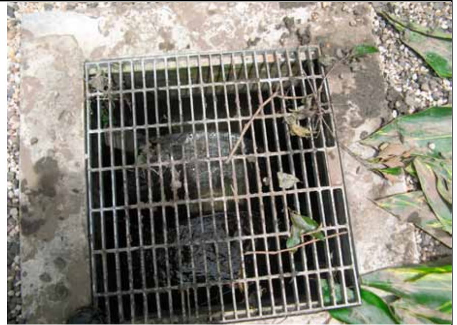
The large grate giving access to the stormwater drain at the side near the footpath gate on 14/01/11 at 1.04 pm, which can drown a person, if they fell in and could not get out
