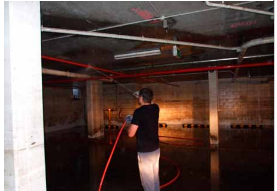
Inside view of one set of vents where water entered Basement 1 carpark
