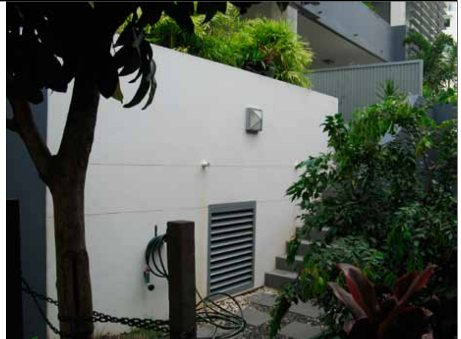
Vents at the back of Aura with the sunken garden below ground level
