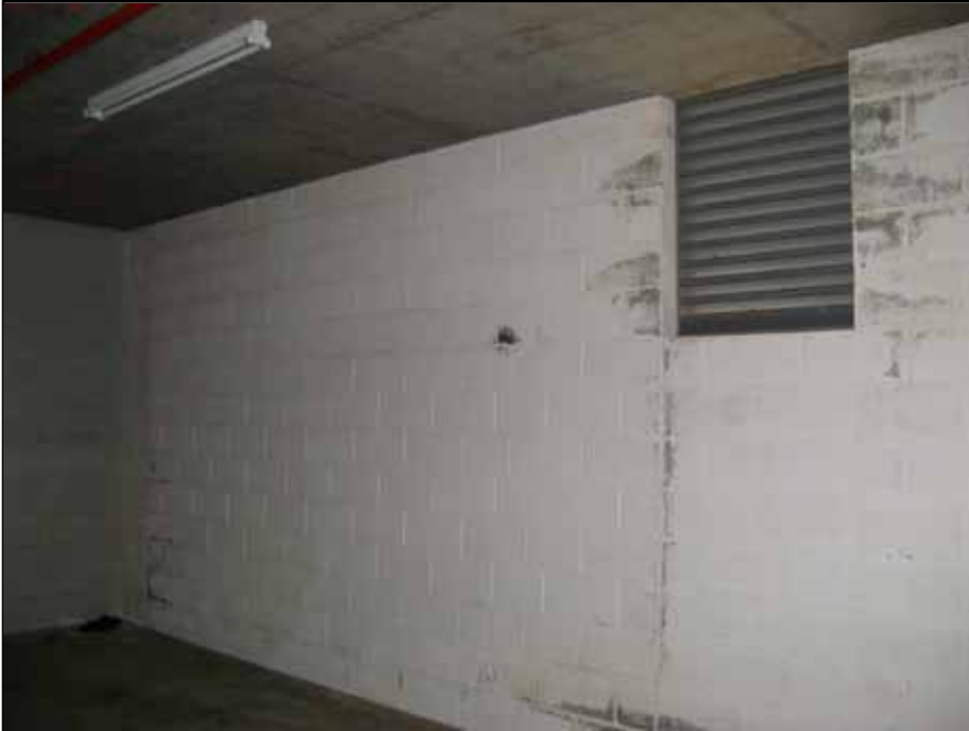
Basement 1 vents where water entered carpark
