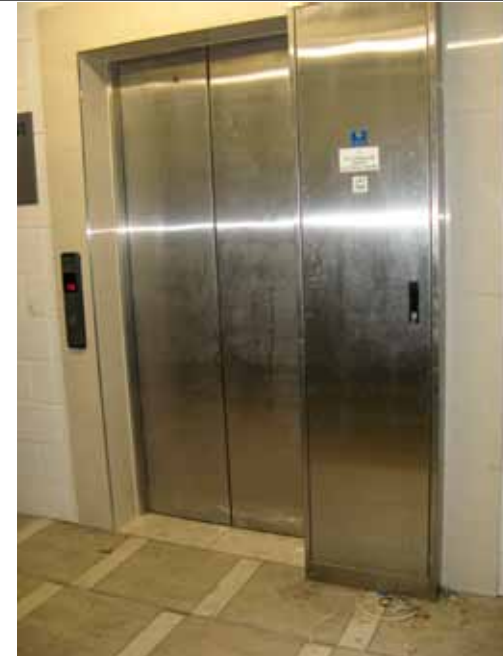
Aura lift doors on Basement 2 with controls on the right
