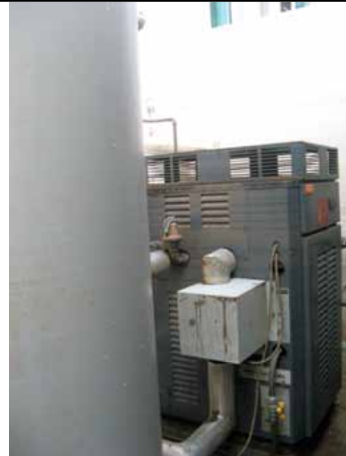
Water heater controls that were completely submerged and damaged by water
