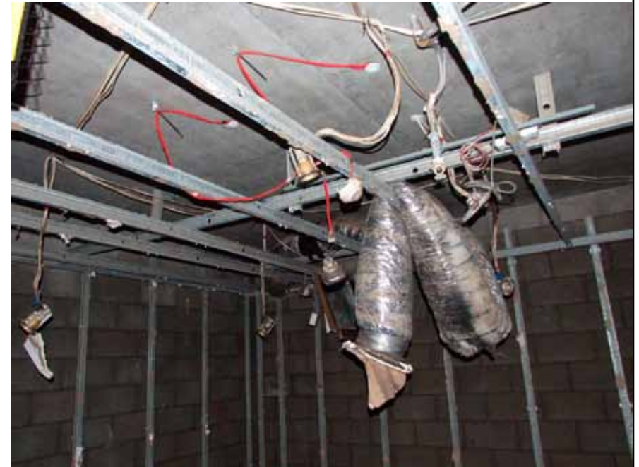
Part of the CO2 ventilation system
