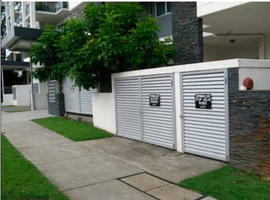
Room on left under tree housing Energex transformer for Arriva & Aura Apartments where water entered
