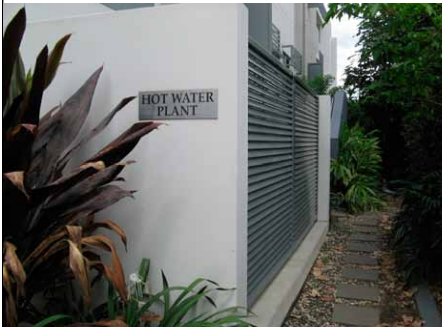
Room housing the water heaters beside the building and well below the building ground floor
