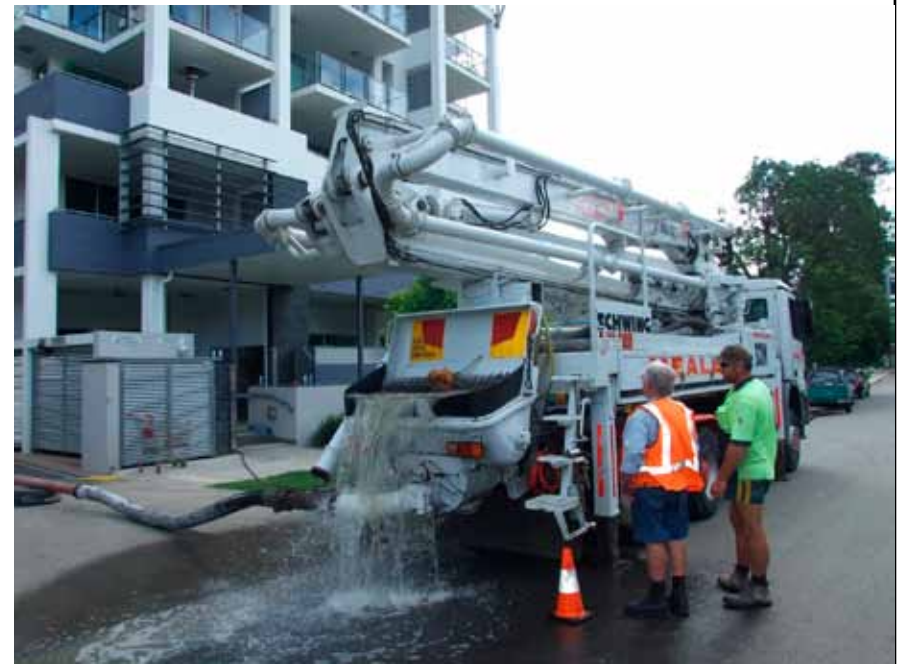
Pump truck needed to pump out Basement 2
