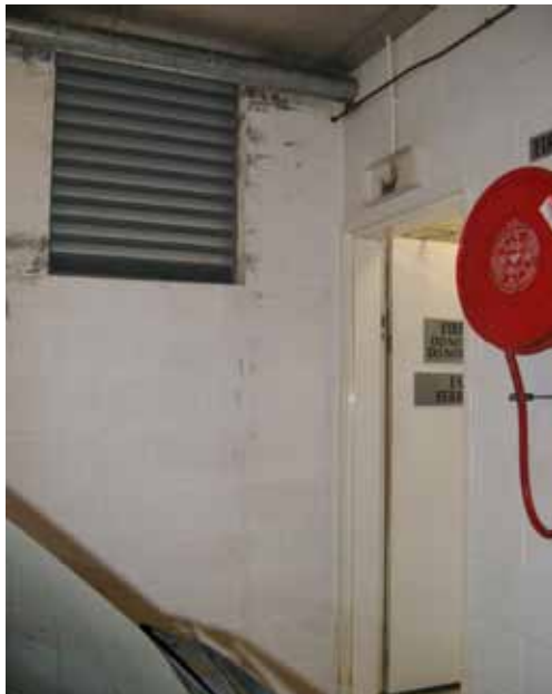
Basement 1 vents where water entered carpark
