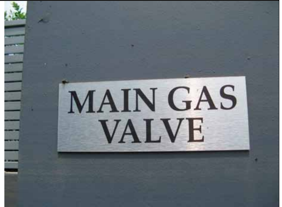
Main gas valve sign beside the stairs to the basements
