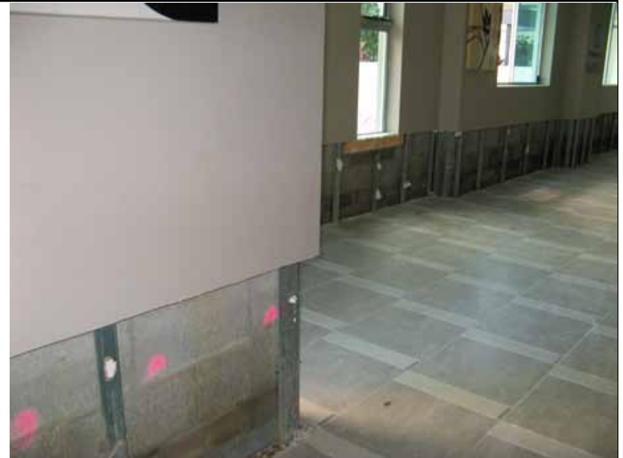
Damaged walls in the Aura foyer
