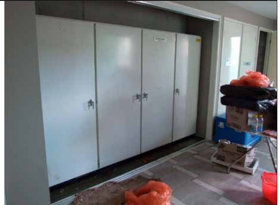
Power control panel inside Aura's foyer where partial damage occurred to the building power distribution.
