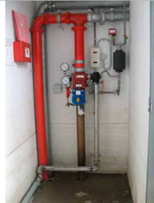
Inside the fire sprinkler system that was damaged by water
