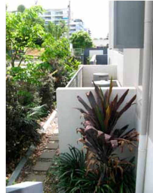
Looking down on the water heaters from the entrance to the fire stairs at ground floor level
