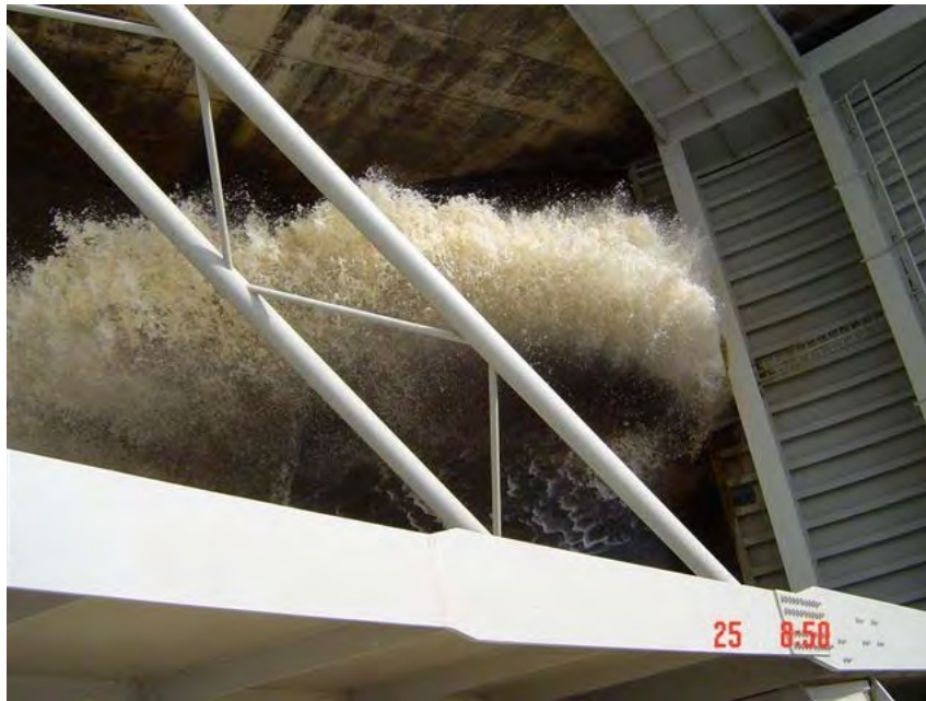
Dam crest seal failure
