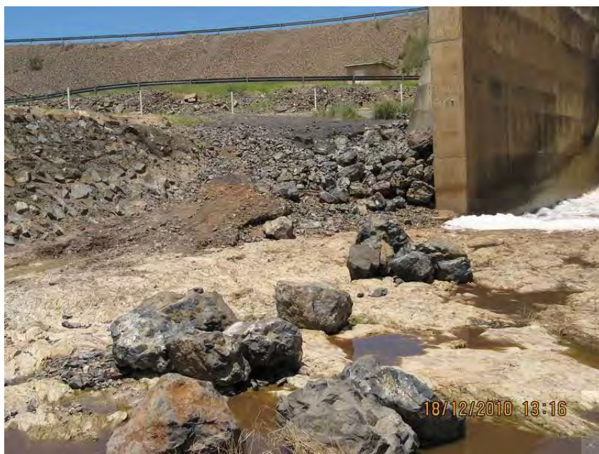
Access ramp to down stream area eroded away
