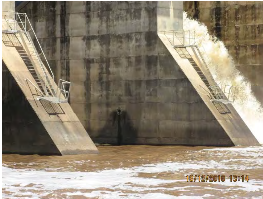
Access service ladders damaged and missing lower ladder, washed away
