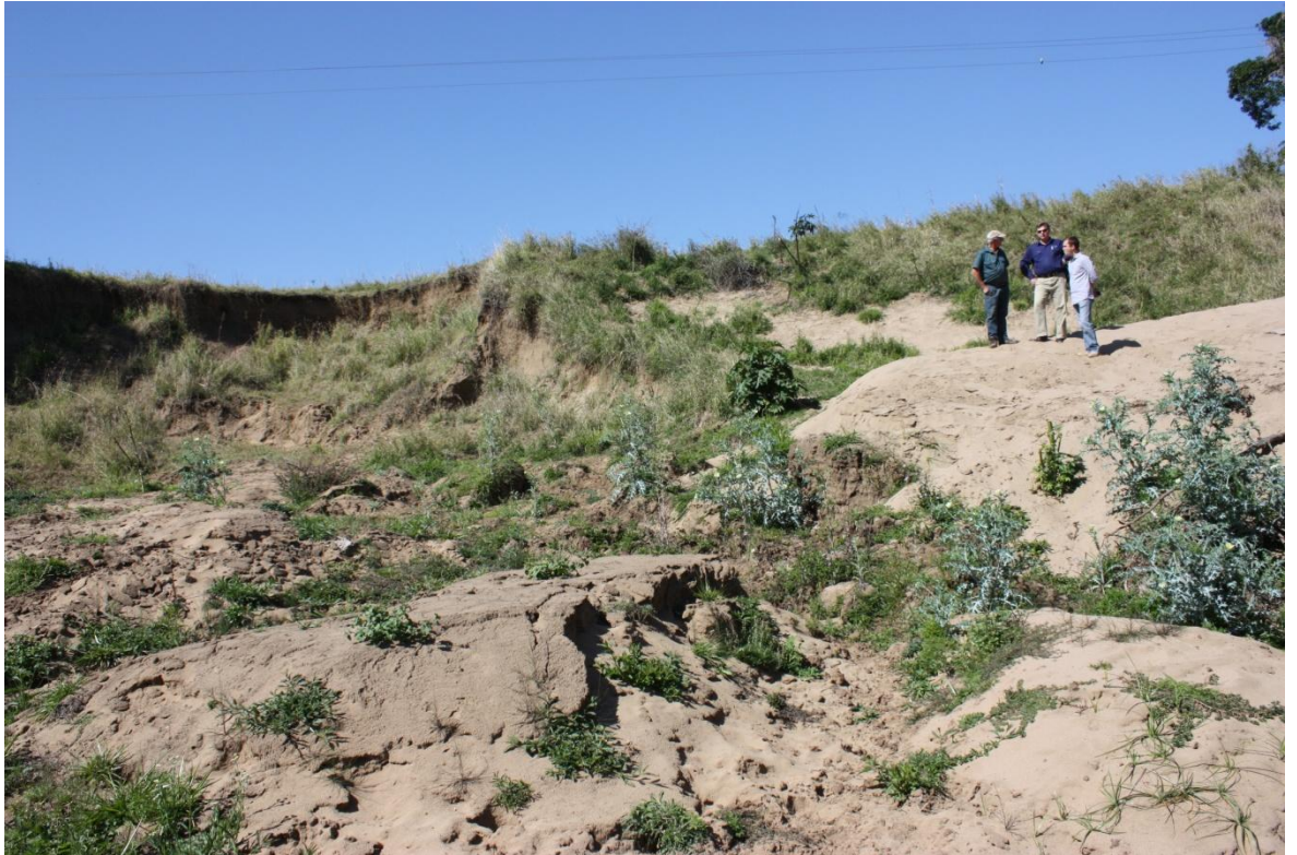
Figure 5: Mass failure of right bank at Fernvale and overbank deposition.
