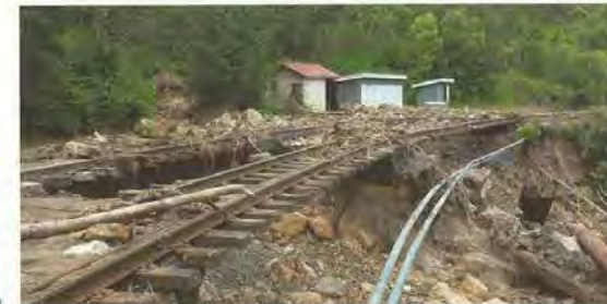
Track damage Spring Bluff
