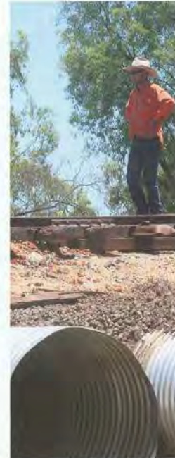
A contractor inspects damaged track in Emerald
