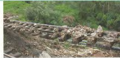
Track damage Spring Bluff
