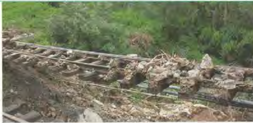
Track damage Spring Bluff
