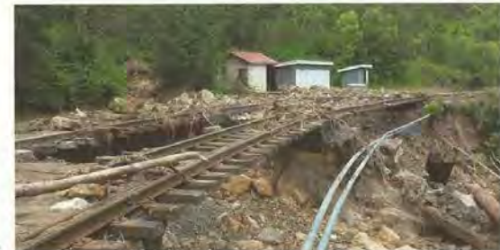
Track damage Spring Bluff
