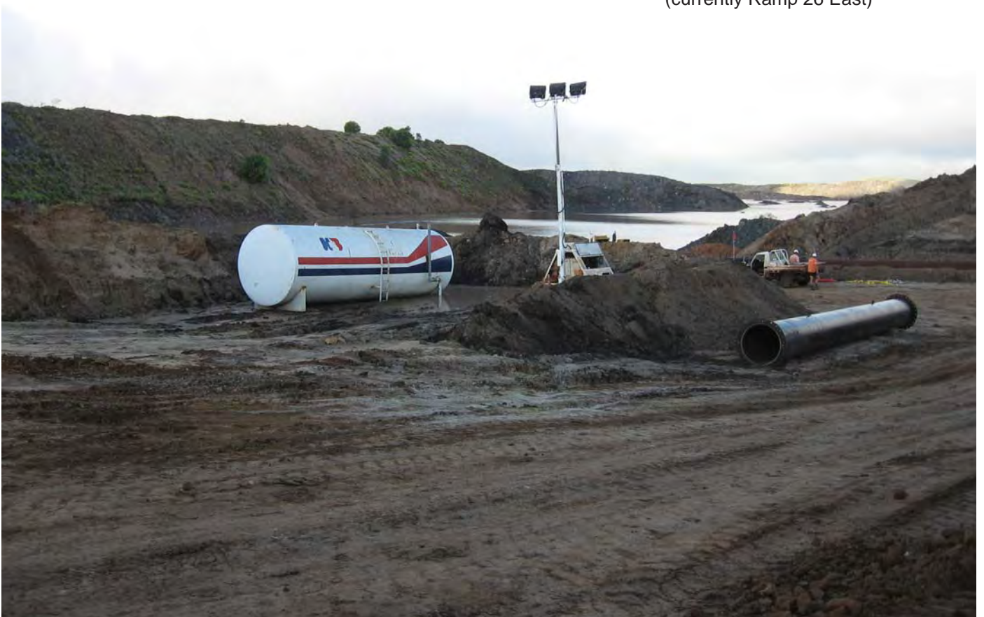
Typical Bunded Pump Fuel Tank Installation (currently Ramp 26 East)
