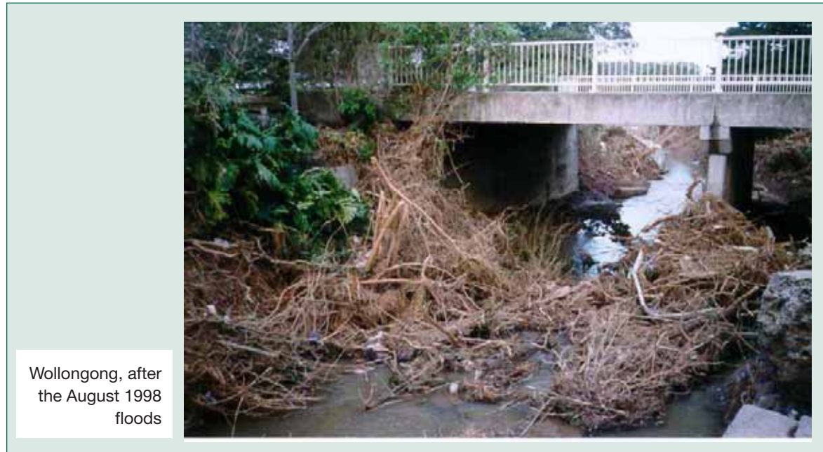
Figure 36 Debris can partially block larger waterways
