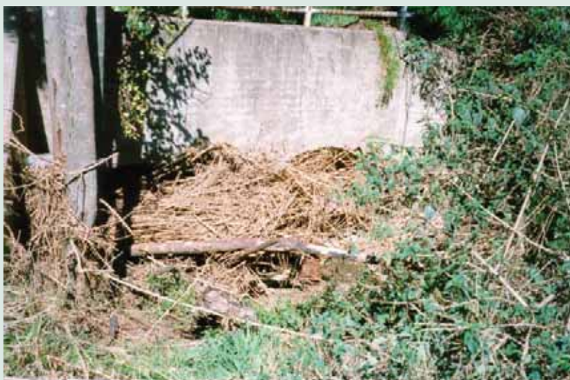
Figure 35 Small culvert openings in highly urbanised areas are easily blocked by debris
