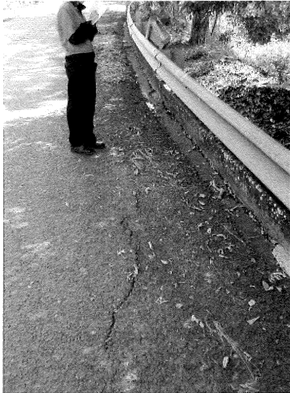
Figure 16: In filled tension crack at Location 2
