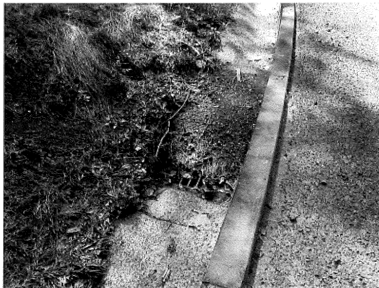
Figure 19: Partially blocked cross drain, located along access road.
