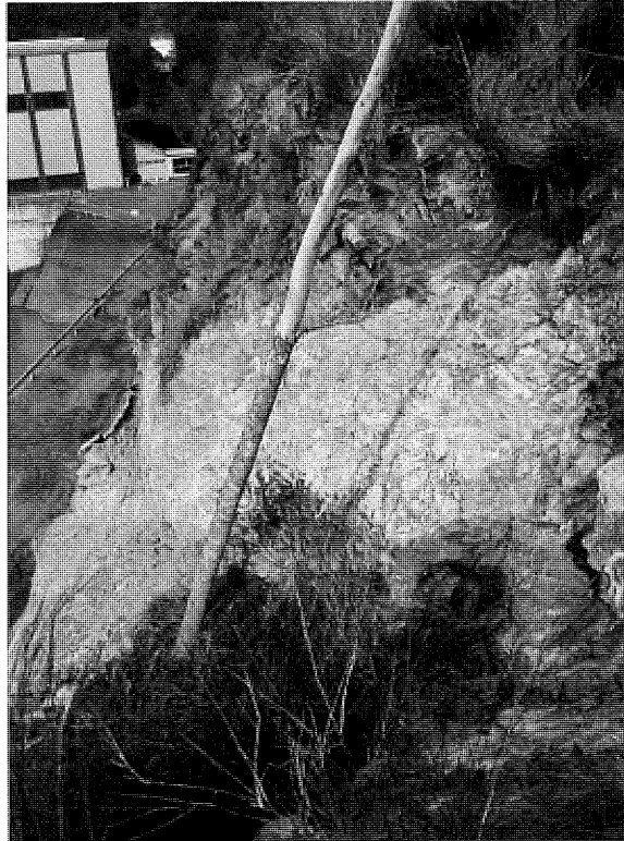
Figure 5: Weathered rock toppling from slope below sewer-line bench.
