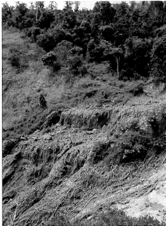
Figure 9: Benched slope behind the power station illustrating degradation and wasting due to overland flow.
