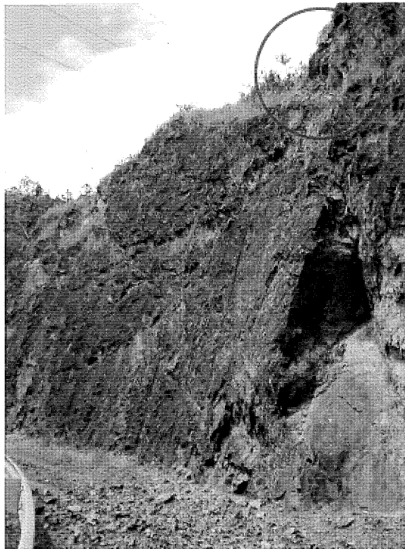
Figure 8: Minor rock fall associated with unfavourable jointing, south-eastern access track area. Note that wedge failure in foreground occurred some years ago.
