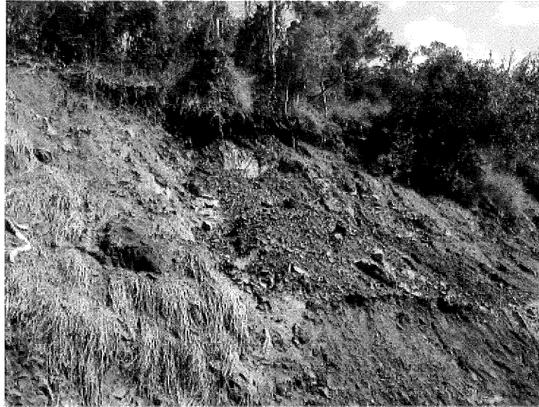
Figure 14: Over slip present in the upper section of the access road.
