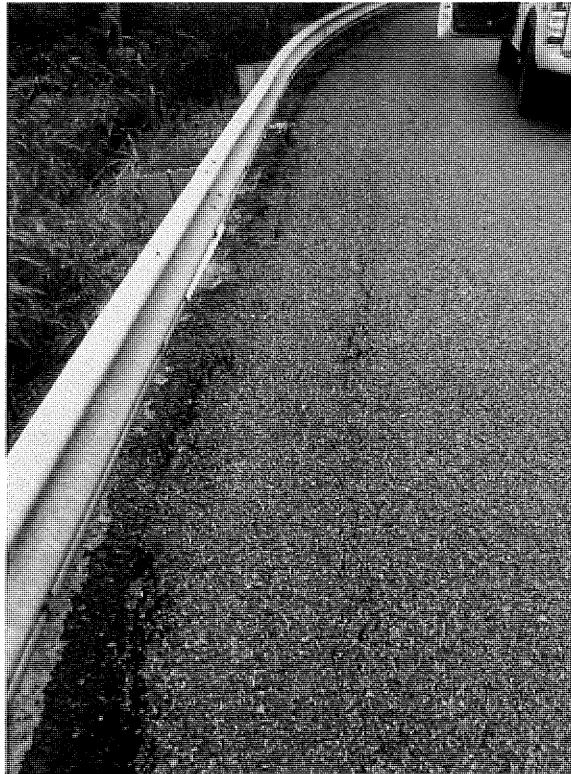
Figure 15: Tension crack and tilted guard rail located approximately 100 m north of the security building (Location 1).
