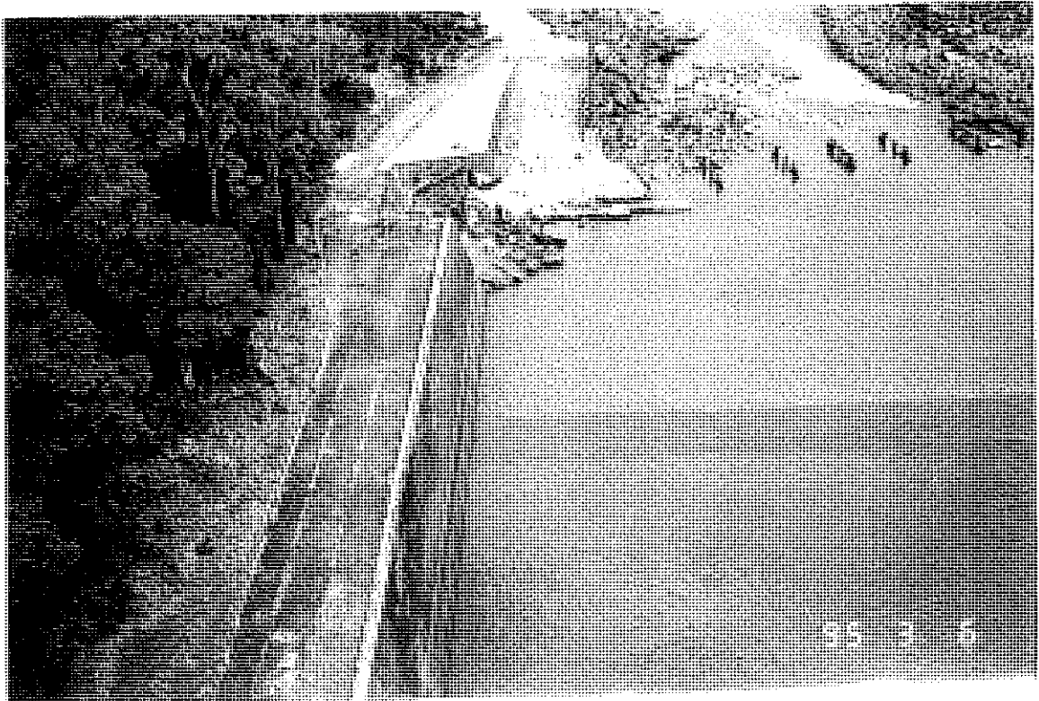
Left Abutment Stilling Basin Wall - Note backfill to full height, no weep holes, grass growing in joints on top sealing slab.
