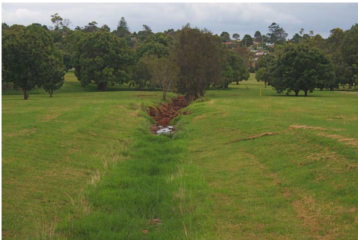
Photo No.2 East Creek at Spring St Looking Downstream: Bank Erosion Along Grassed Waterway
