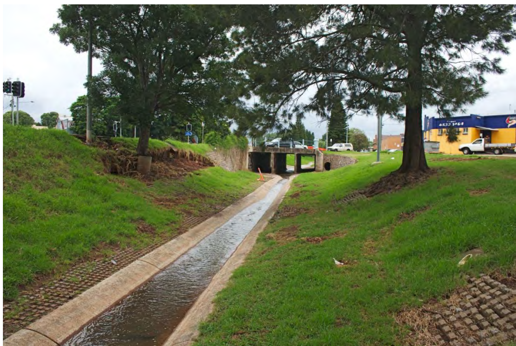
Photo No. 4 East Creek Looking US at Neil St Culverts: Grassed Waterway with Concrete Low Flow Channel, Erosion on RH Bank, Depth of Flooding 1.5-2 m above Neil St
