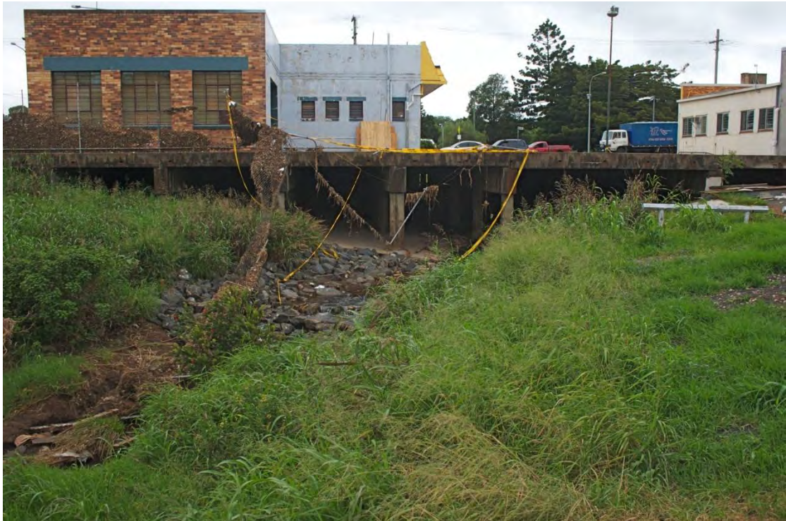
Photo No. 5 East Creek Outlet Under Ruthven St: Note Flood Debris on Fence; Floodwaters were some 2m Above Deck Level
