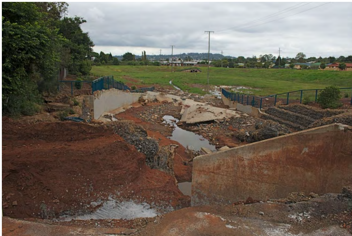
Photo No. 8 West Creek at James St Looking Downstream into James St Detention Basin: Outlet Works Under James St Destroyed.
