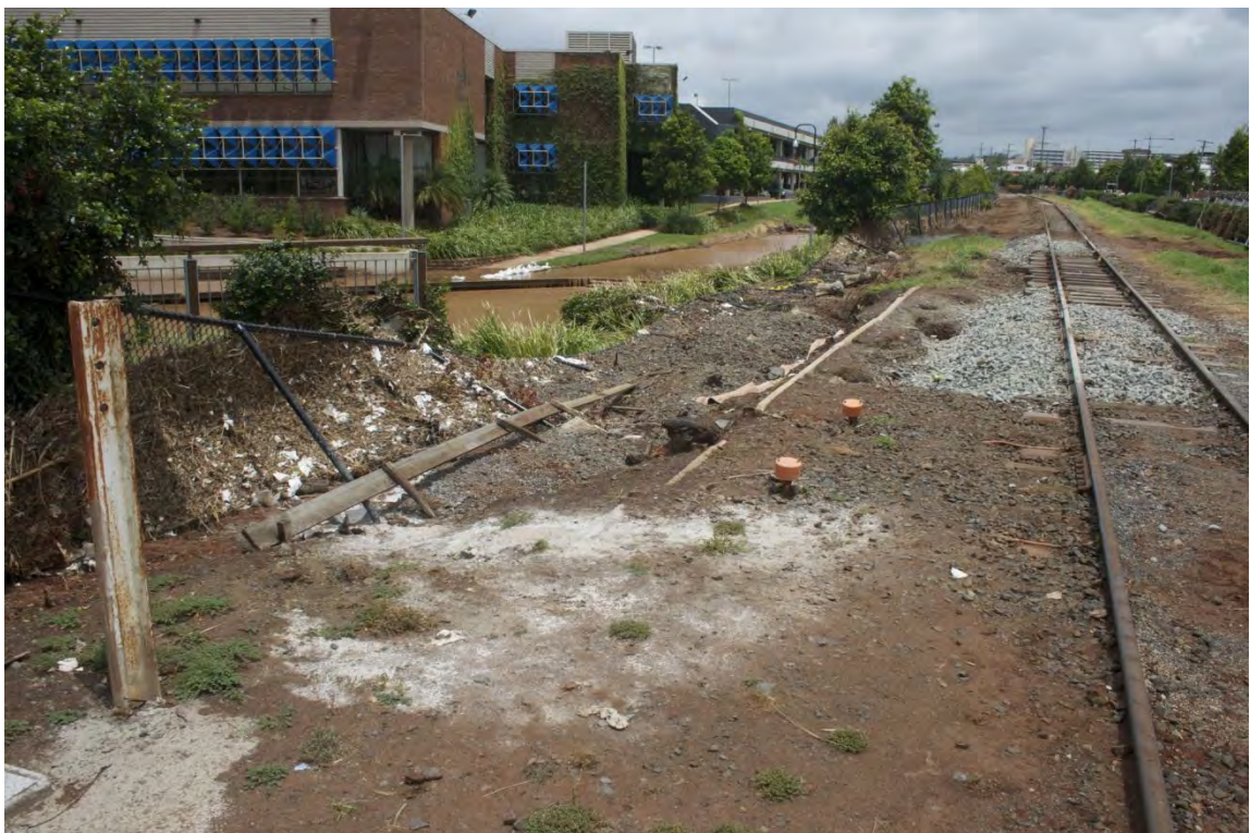
Photo No. 10 Looking South Along Railway Line Opposite Dent St, West Creek to LHS: Easterly Flowing Floodwaters that Overtopped the Embankment Destroyed Fence When Returning to West Creek
