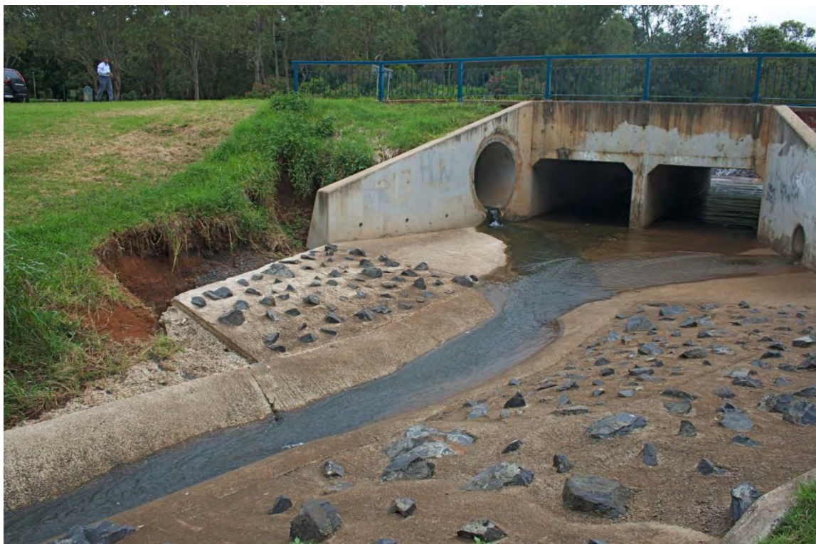
Photo No. 6 West Creek at Spring St, Looking Upstream: Spring St overtopped by 0.5-1 m, Erosion on RH Bank Caused by Floodwaters Overtopping Road
