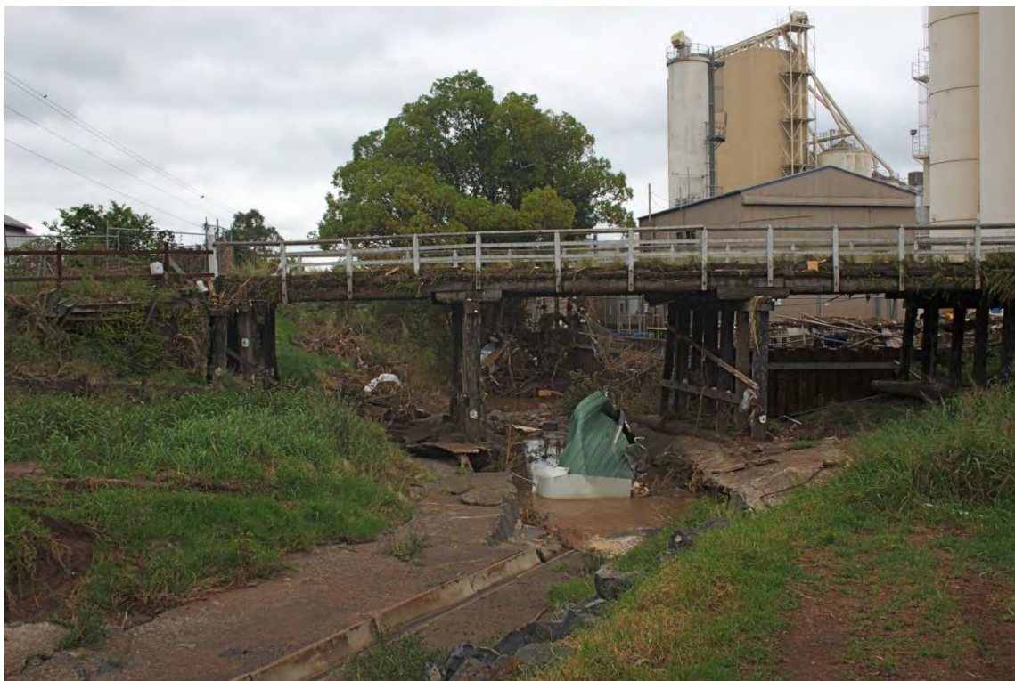
Photo No. 13 Disused Bridge Immediately DS of Junction of East and West Creeks (Flour Mill in Background): Floodwaters 1.5-2 m Above Deck Level of Bridge, Flood Debris Readily Apparent in Creek.
