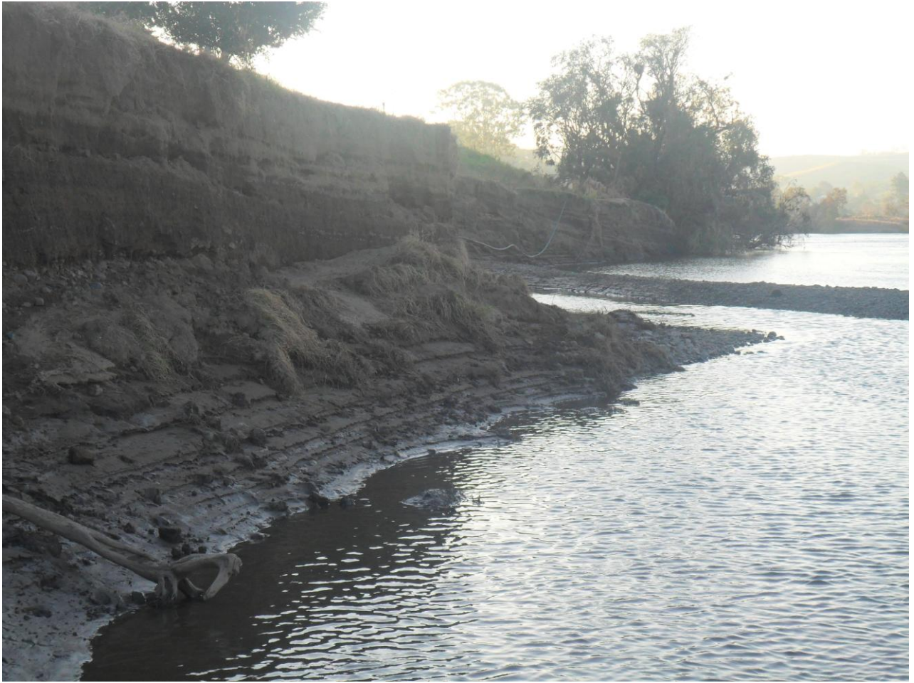
04. Exposed and unstable banks
