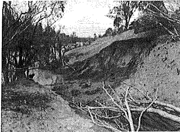
Photo 005 – Jan 11 Pump Site Riverbank Slump Beginning
